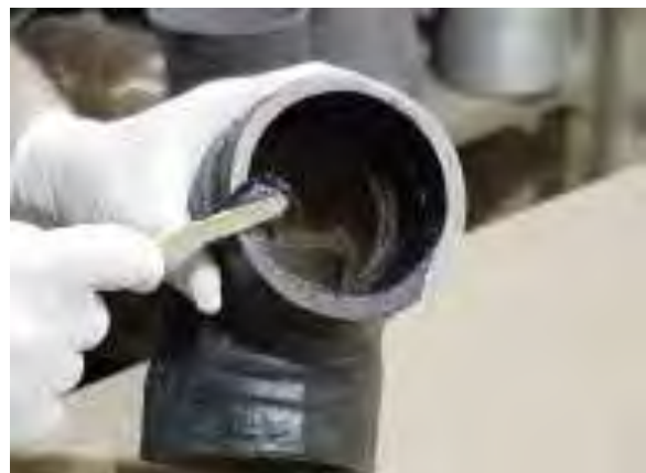
Figure 11 Seal face of the fitting
